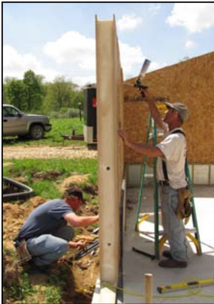
B&K Construction installs Structural Insulated Panels for the Fontana Cabins. The SIPs provide better insulation and less air infiltration compared to conventional walls.
