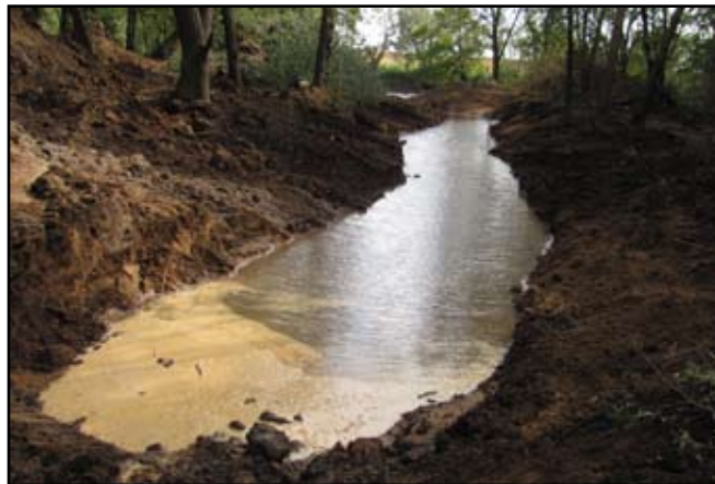
A channel was dug in late summer at Cortright Wildlife Area. The project reconnects wetland ponds to the Wapsipinicon River.
