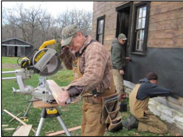
A grant from the Buchanan County Community Foundation provided material for replacing siding on the historic Richardson-Jakway House. Don Shonka (above) was one of several volunteers who assisted staff in replacing the siding.
